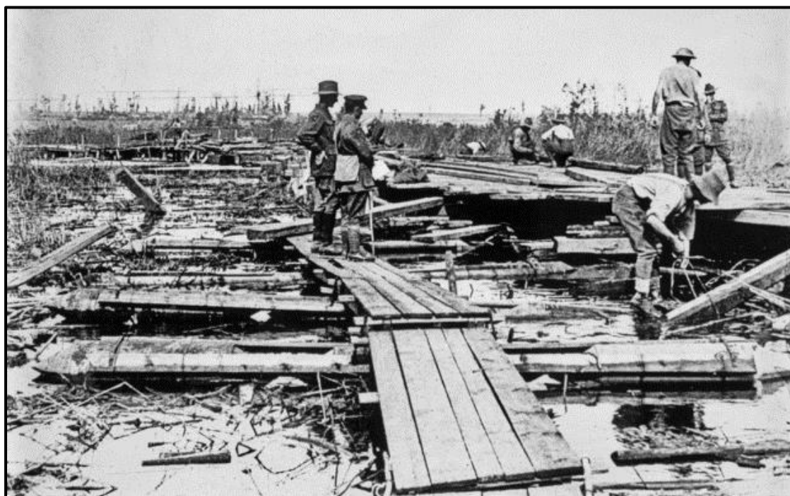
Engineers erected pontoon bridges across marshes and rivers prior to an attack (Australian War Memorial AWM A01908)
